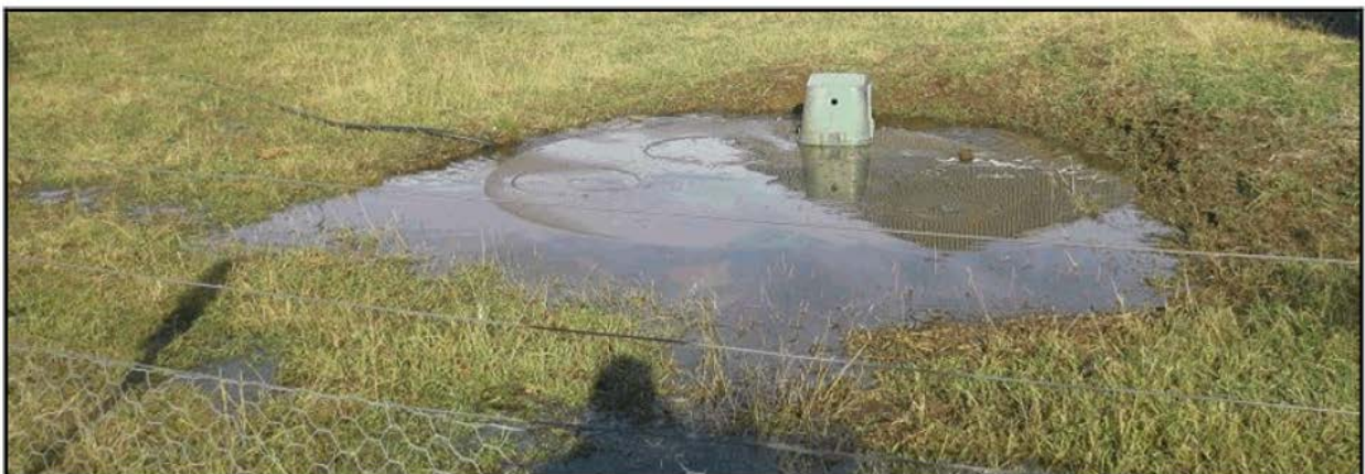
Figure 5: Inundated Septic System (Planning for Gundaroo, December 2014)
